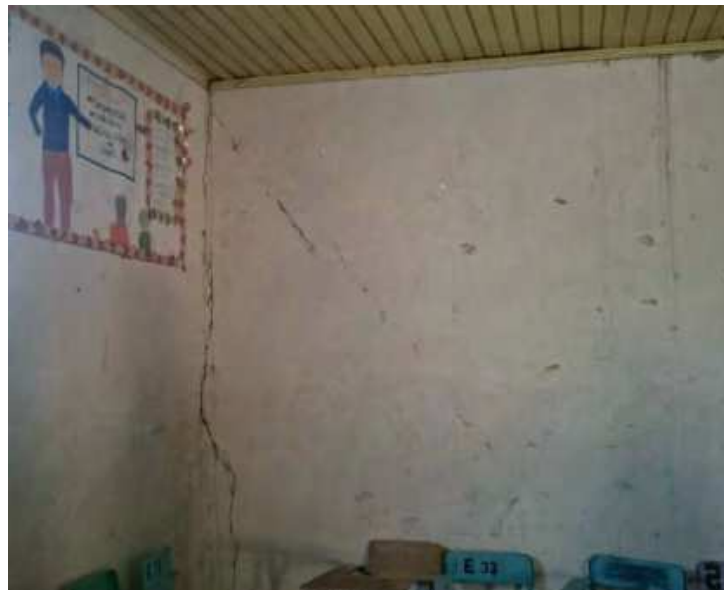
Figure 20 – In-place cracking of URM
