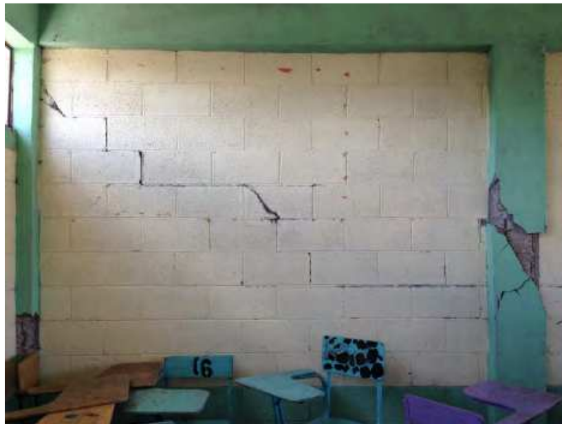
Figure 22 – In-plane shear failure (masonry and column)
