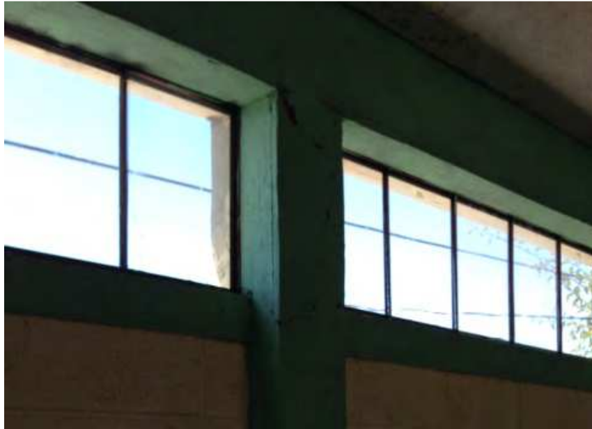
Figure 23 – Short column shear failure damage
