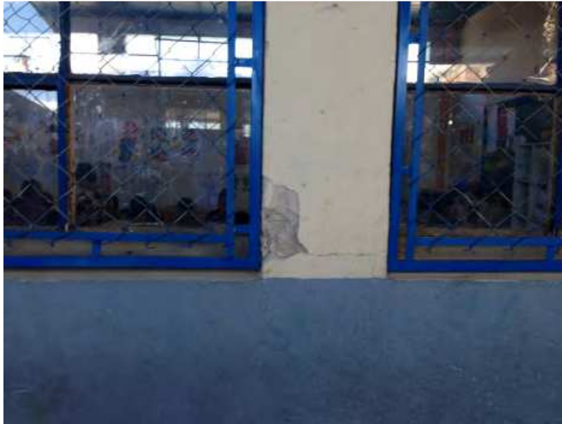
Figure 30 – Cracking at column base at window sill
