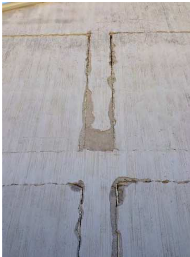
Figure 14 – Significant panel edge cracking
