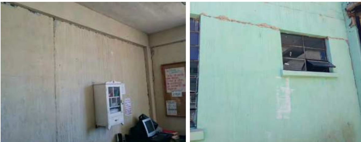
Figure 12 – Cracking around infill panel perimeter at interface with concrete frame at interior (left) and exterior (right)
