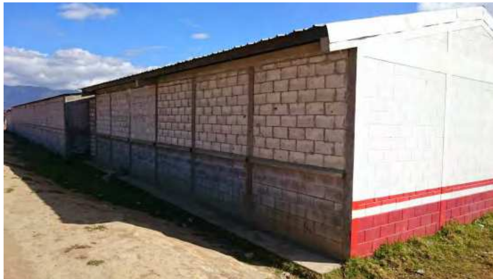
Figure 37 – Masonry infill at damaged classroom windows
