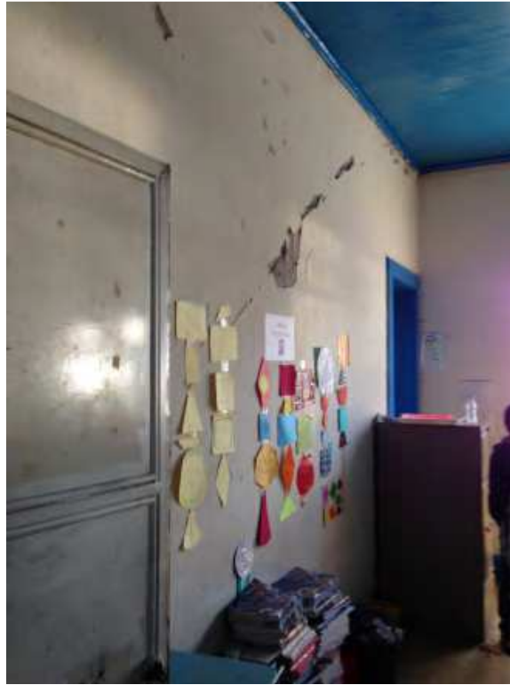
Figure 32 – Shear cracking in wall panels
