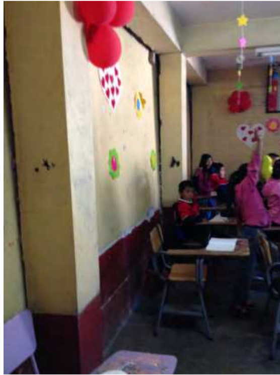
Figure 25 – Out-of-plane wall movement and separation from frame
