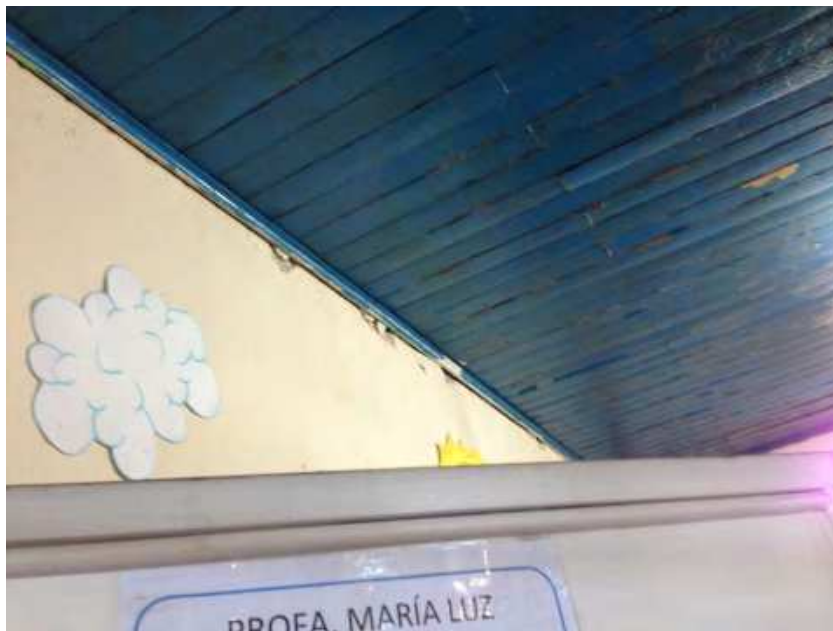
Figure 31 – Cracking at the top of walls (where wall and ceiling pulled apart)
