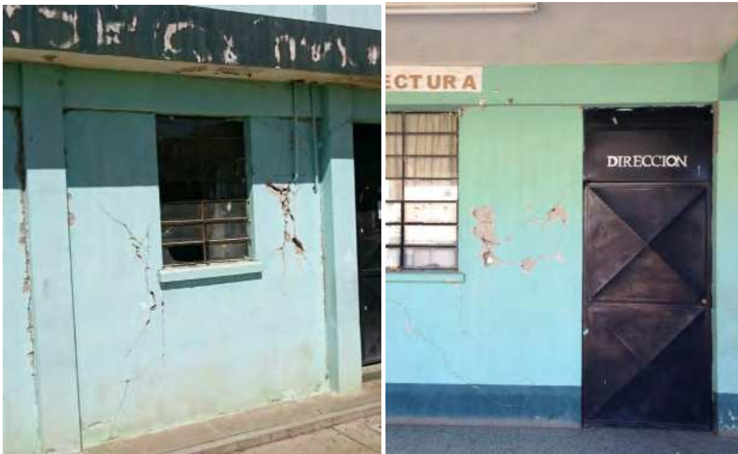
Figure 16 – Shear cracking of infill
