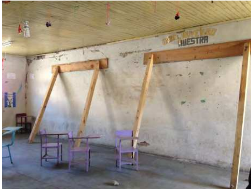
Figure 21 – Unreinforced masonry wall out-of-plane failure
