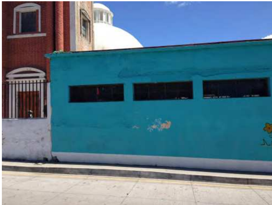
Figure 29 – Evidence of horizontal cracking at wall-roof intersection
