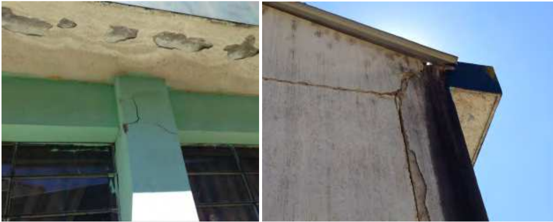
Figure 13 – Column-to-beam joint damage
