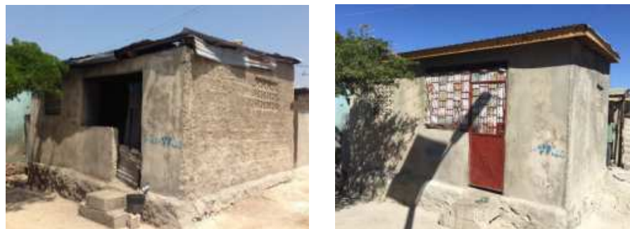
Figura 3: A home in Port-au-Prince before (left) and after (right) a seismic retrofit
