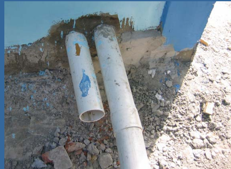
Bad Practice (Buruk) Graywater draining into foundation
