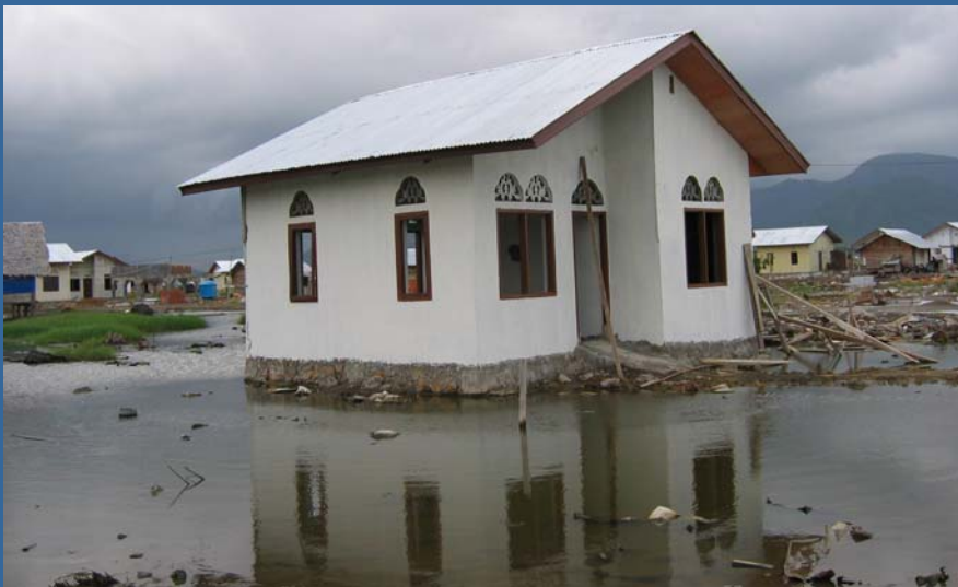
Bad Practice (Buruk) No drainage
