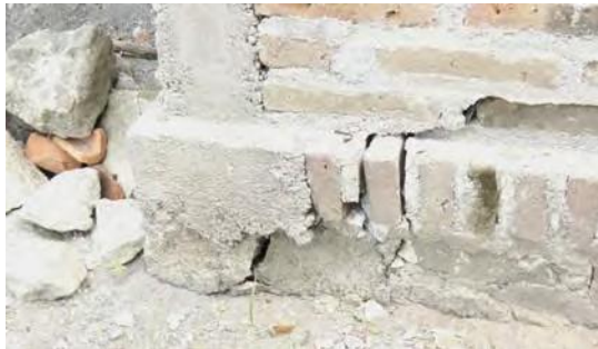
Figure 25. Displacement along wall/foundation interface, Tegal Kebong Agung, Imogir (Bantul) S7.93434° E110.36667°, CIMG1769
