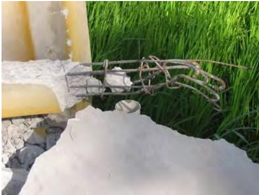
Figure 18. Connection failure, RC frame building, Central Java
