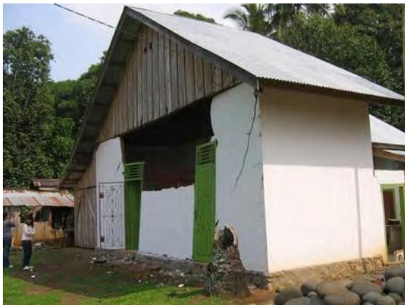
Figure 11. Confined masonry building with overturning failure of tall, unsupported wall, Kec. Airnapal (North Bengkulu)
