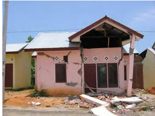
Figure 14. Subdivision of confined masonry houses, damage to covered terrace, Bengkulu. S3.83218° E102.29287
