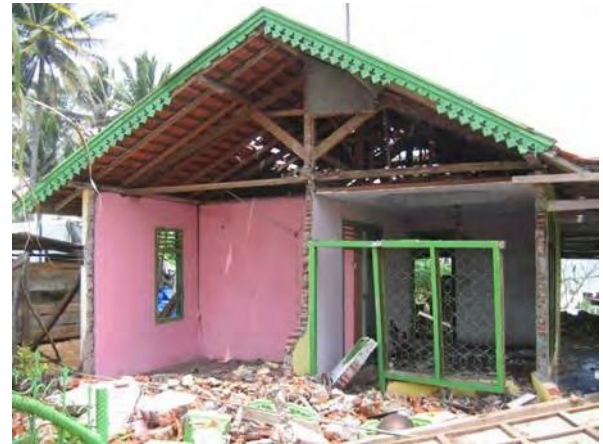
Figure 9. Partially collapsed brick masonry house with RC tie columns and timber bond beams, note partial collapse of masonry gable wall, and lack of in-plane stiffness in front wall, Kec. Lais (North Bengkulu) S3.53217° E102.03771
