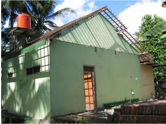
Figure 4. Masonry gable wall overturning in 27 May 2006 Central Java Earthquake, Keputren, Pleret (Bantul) S7.86905° E110.40272°, IMG_6721
