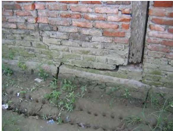
Figure 26. Cracks in foundation and walls associated with settlement and tilt on liquefiable soils, Lempuing (Bengkulu), S3.82799° E102.28473
