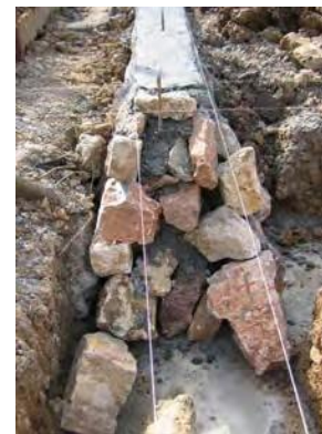
Figure 11. Poorly built stone masonry strip footing. Note gaps between stones, stones standing on end.
