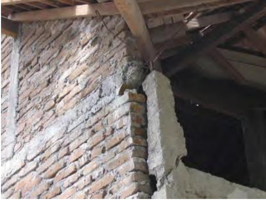
Figure 19. Insufficient connection between wall and tie column and between tie column and bond beam, Pleret (Bantul) S7.88174° E100.40869°, IMG_6746
