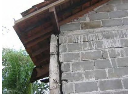
Figure 20. Insufficient connection between wall and tie column and between tie column and bond beam, Segoroyoso, Pleret (Bantul) S7.88174° E100.40869°, IMG_6749
