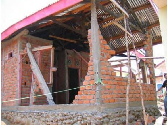
Figure 21. Subdivision of confined masonry houses, collapse of masonry wall exacerbated by insufficient connections, Bengkulu. S3.83218° E102.29287
