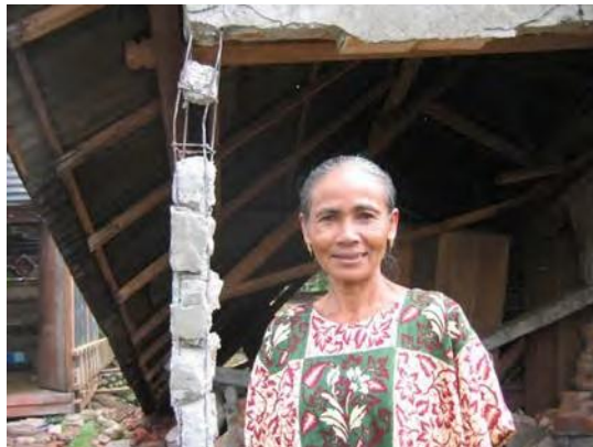
Figure 24. Homeowner standing in front of her collapsed wall, note quality of concrete, Padang Panjang, IMG_8840.
