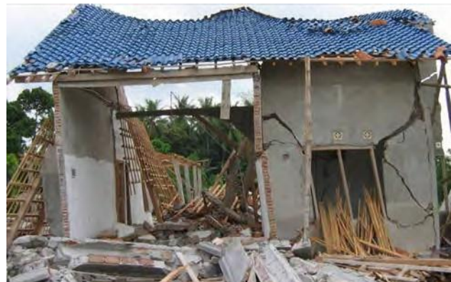
Fig. 3. Confined masonry house under construction, insufficient connections, Pleret (Bantul). S7.87574°, E110.40703°, IMG_6575
