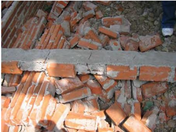
Figure 23. Close up view of collapsed ring beam and wall, same as Fig. 20. Failure plane between top of mortar bed and bottom of brick above it.
