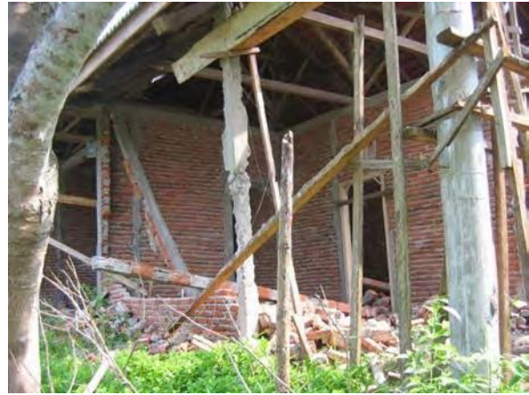
Figure 22. Confined masonry house with failure in masonry walls and connections between tie columns and bond beams, Kec. Airnupal (North Bengkulu)
