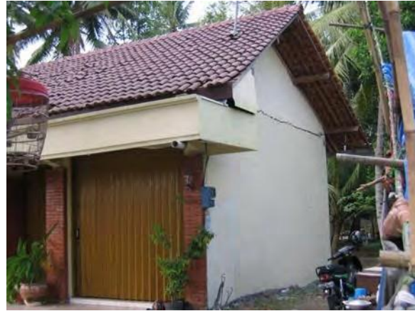
Figure 5. Masonry gable wall overturning in 27 May 2006 Central Java Earthquake, (Bantul) S7.89468°, E110.37341°, IMG_6542
