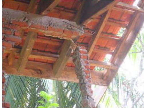
Figure 17. Confined masonry house with failure in masonry walls and connections between tie columns and bond beams, Kec. Airnapal (North Bengkulu)
