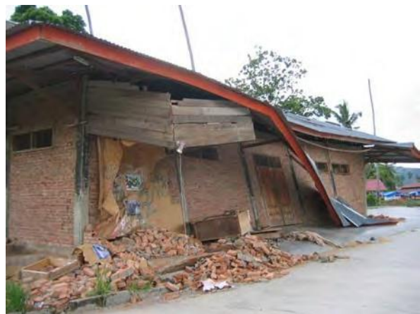
Figure 12. Confined masonry warehouse with overturning failure of long walls without cross-bracing, , IMG 8891
