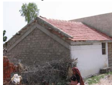
Fig. 1. Missing gable band, seismic belt added (Bhuj EQ)
