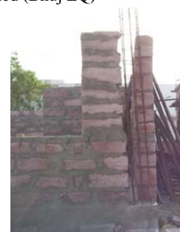
Fig. 2. Confined masonry under construction, note large openings, wide gap between stone and rebar, rebar out of plumb (Bhuj)
