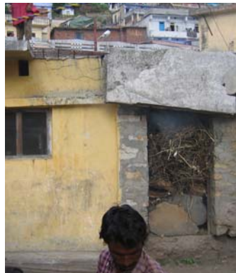
Fig. 3. Partially collapsed, newly built RC slab roof (Chamoli EQ)
