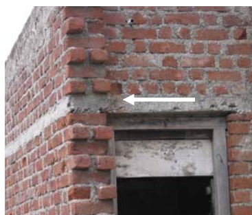
Fig. 6. Masonry bond for extension; short rebar length (Killari EO)
