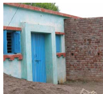
Fig. 7. Extension without proper connection (Killari EO)
