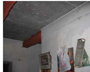
Fig. 4. Precast plank and joist system with crack along joist-wall interface, leakage between planks (Chamoli EQ)
